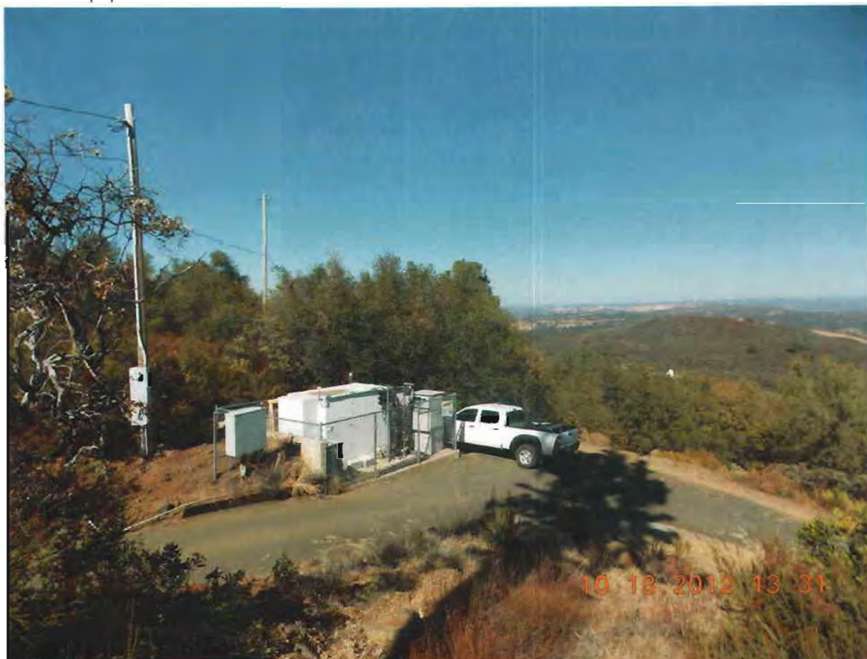
Ground equipment and access road
